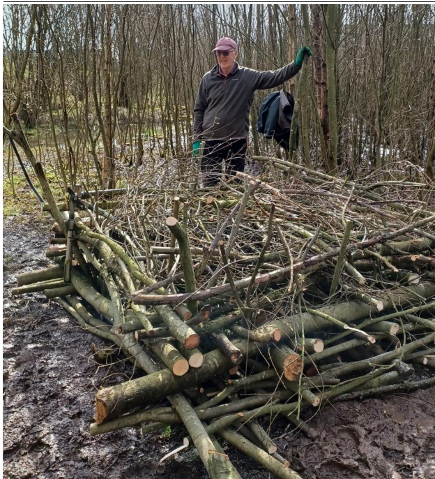
Construction of one of the new Fen viewing area refuges in progress (photograph by Lesley Walker).
